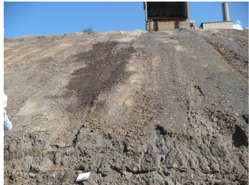
BAP #8 – seepage-interior slope of north dike
